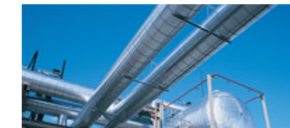
Advising IVG Caverns on the expansion of cavern fields in Etzel
