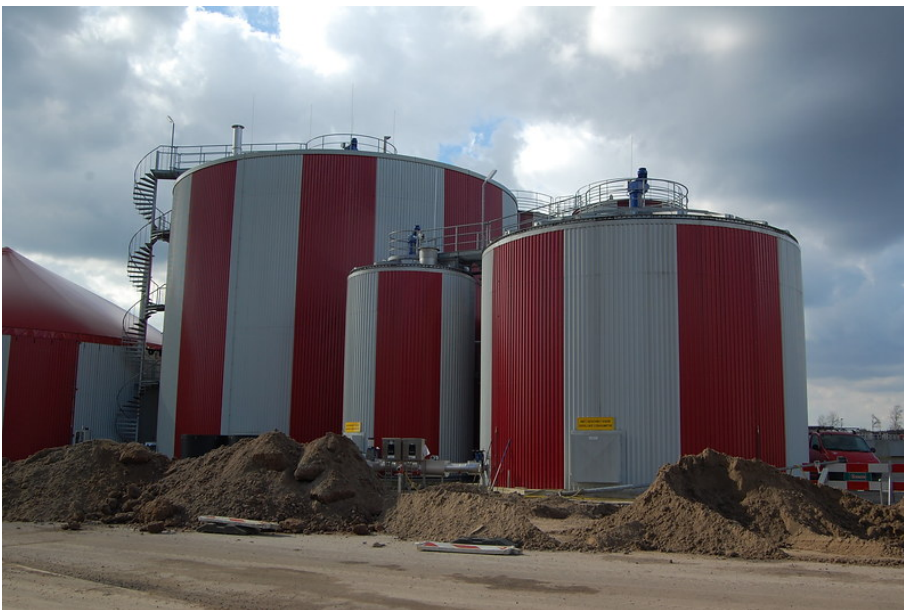
Figure 1 Apeldoorn WWTP, digester tanks
