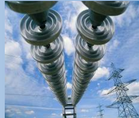
Energy transport, Belgium
